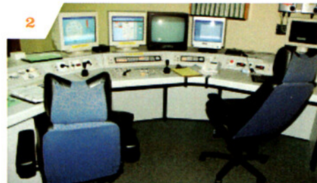
1 Charge machine control room - original layout
