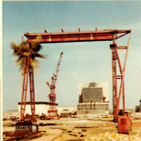
It's needed no more! The crane was brought down by a strategically placed explosive charge.
