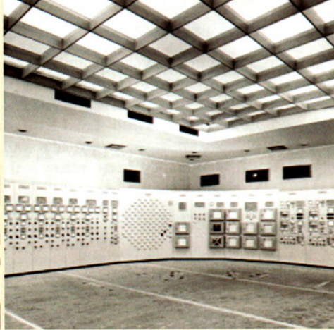
Reactor Two control panel in a strangely deserted Central Control Room. March 1964.
