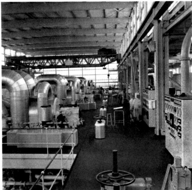
General view of the Turbine Hall.
