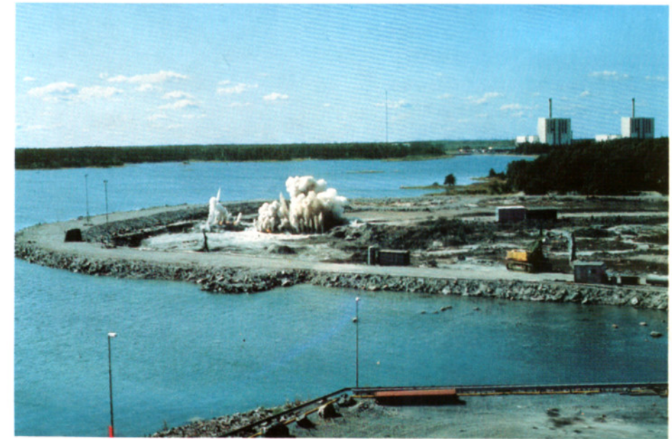
Blasting work for the entrance tunnels to the SFR began in August 1983. In the beginning of 1985 the two tunnels reached the storage area one kilometre outside the harbour at Forsmark.
