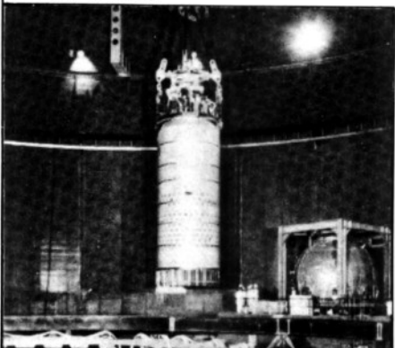
Superphenix : August 1982, installation of the last main component of the reactor block (Core Cover Plug).
