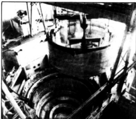
Superphenix : November 5, 1980, installation of the inner vessel (610 tonnes) in the reactor building.
