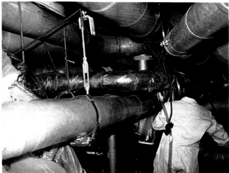
The section of repaired pipe (in polythene wrapping) being replaced preparatory to welding.
